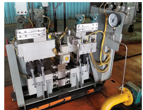
Low pressure example of an on-line testable and repairable hydraulic trip system designed and manufactured by CASE RMC.
